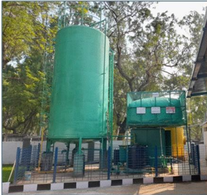
750 kg/day capacity food waste biogas plant Replaces 40 kg LPG equivalent/day Akshaya Patra, Puducherry
