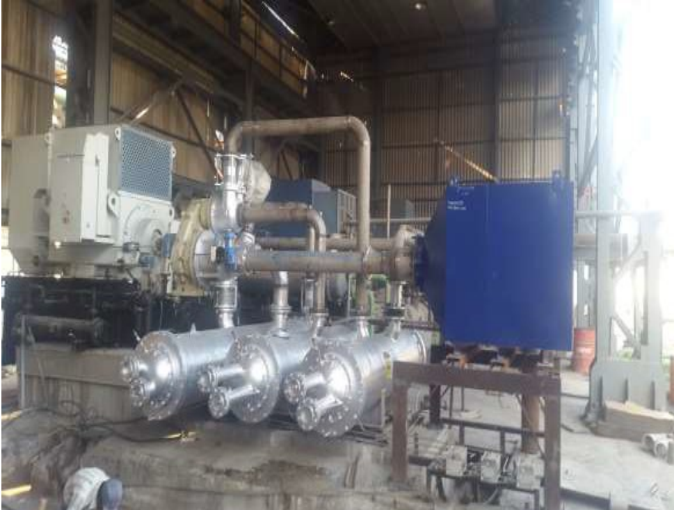
Supply of SS Heat Exchangers to GNFC(Bharuch)
