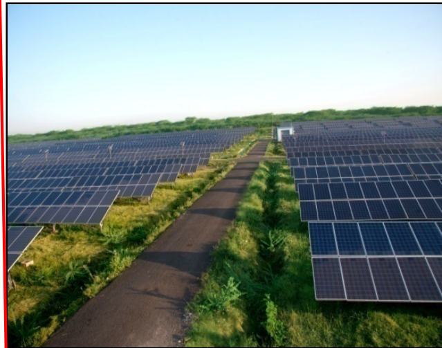
5 MW Solar Plant at SLPP (2012) 2x1 MW Distributed Solar Power cum Agriculture Pilot Projects-2016 TOTAL SOLAR: 162 MW
