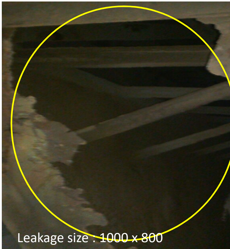
Leakages at Hopper Area
