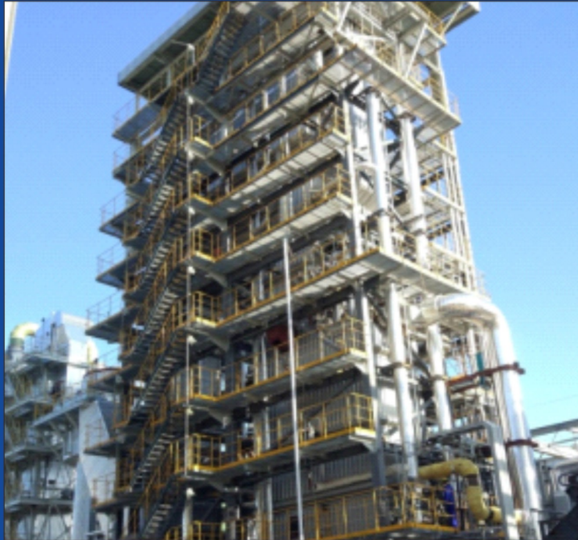
Waste Alkali Incineration Boiler in Shandong NHU Amino Acid Co., Ltd
