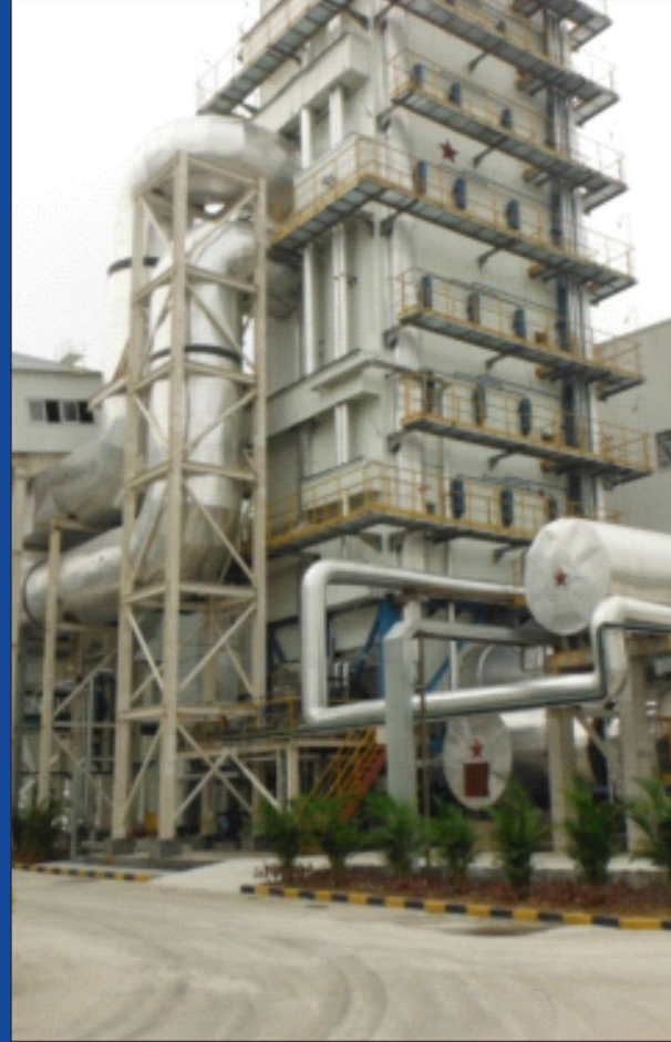
▼ Waste Heat Recovery Boiler for Dongguan CSG900t/d Glass Line
