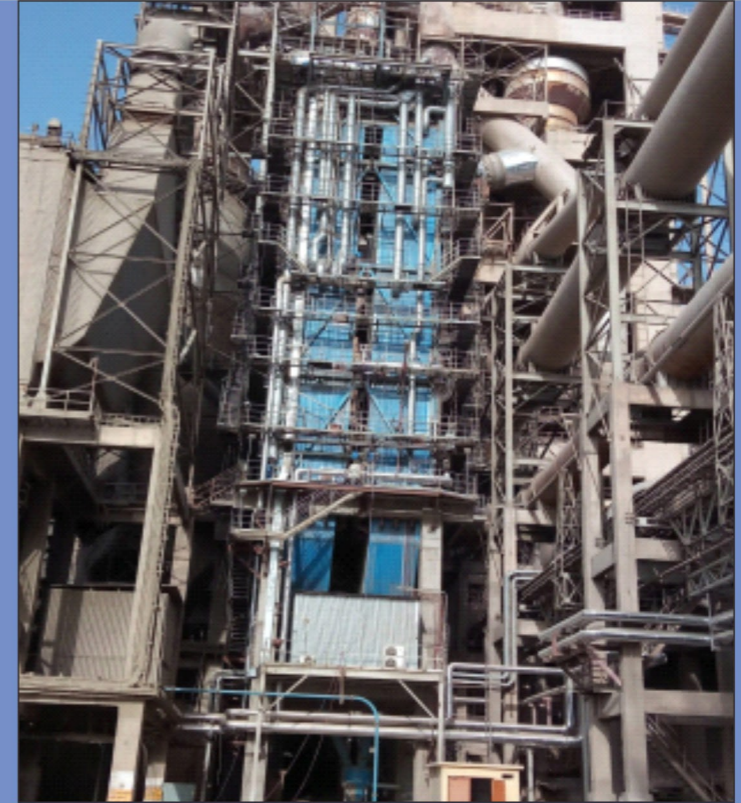
▼ Alkali Bypass Boiler
