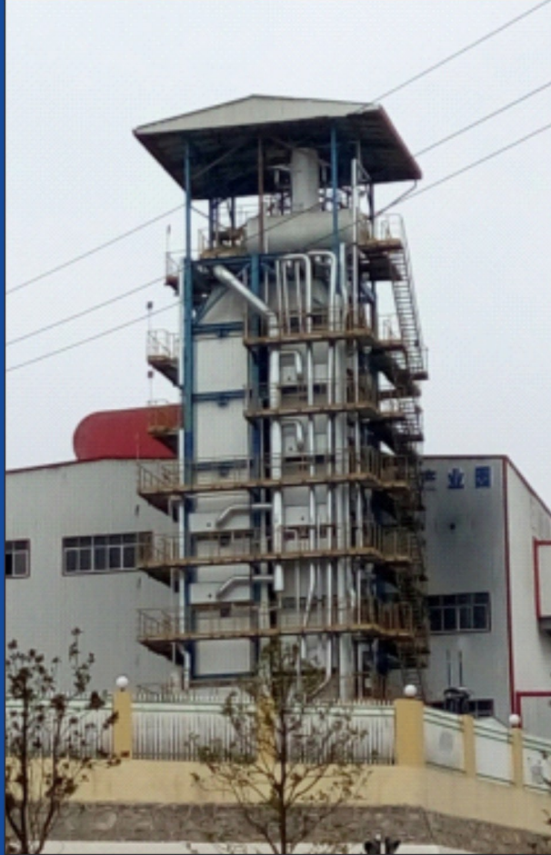
▼ Waste Heat Recovery Boiler for Nanning Fufa 600 t/d Glass Line
