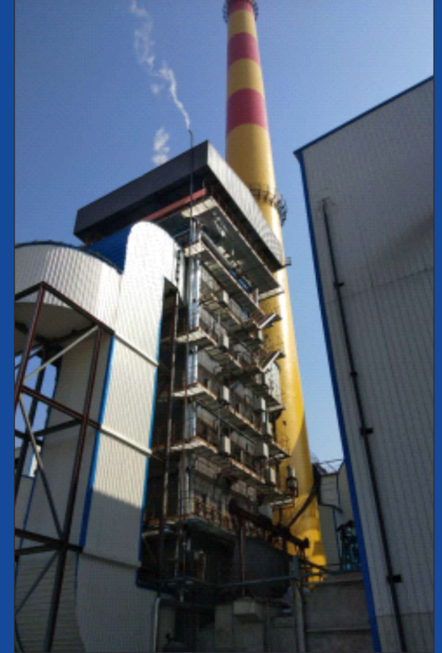
▼ Waste Heat Recovery Boiler for Wuhan Changli 1200t/d Glass Line
