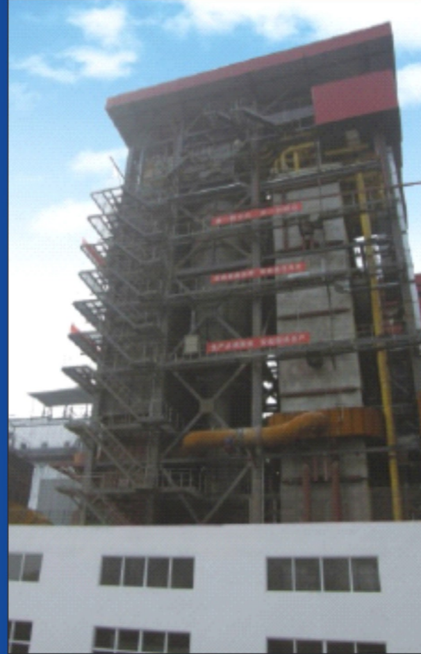
▼ 50 t/hCFB Boiler in Chongqing Chuanran Energy
