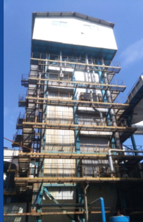
▼ Waste Heat Recovery Boiler for Weihai CSG 900t/d Glass Line
