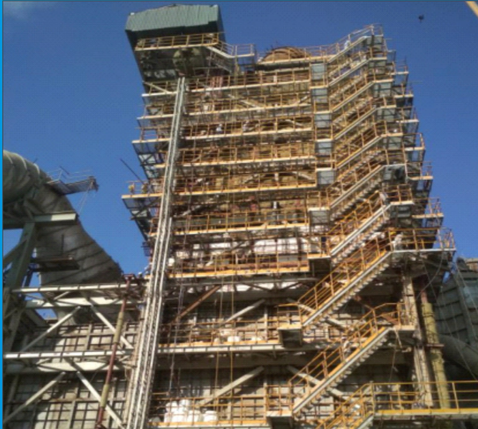
WHR Boiler for Beawar Line-2 5000 TPD Cement Kiln Shree Cement Limited, India
