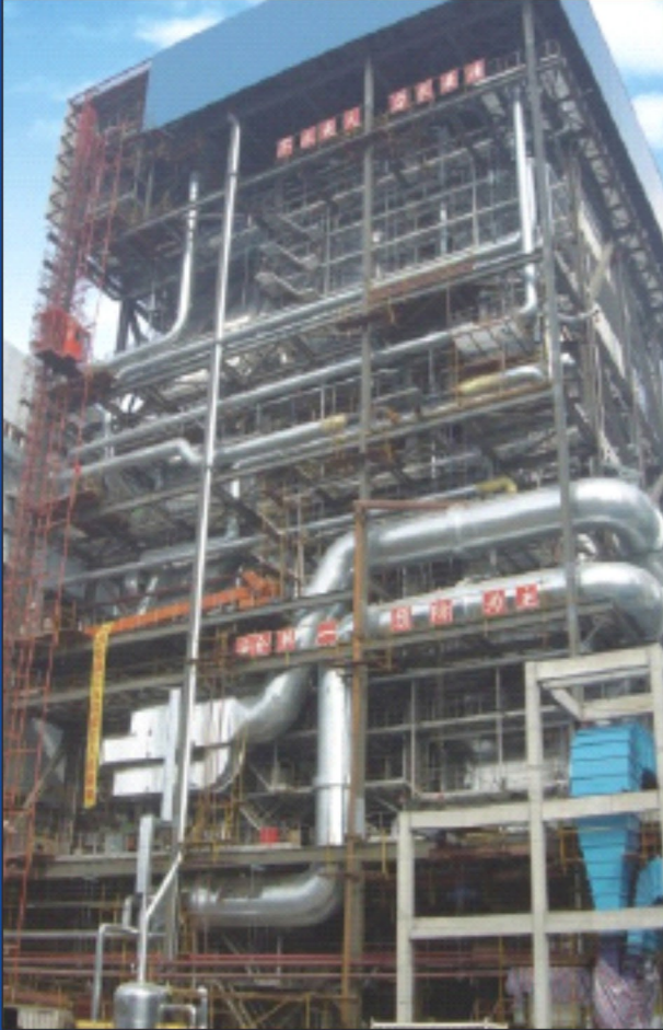
▼ 60 t/hCFB Boiler in Ordos
