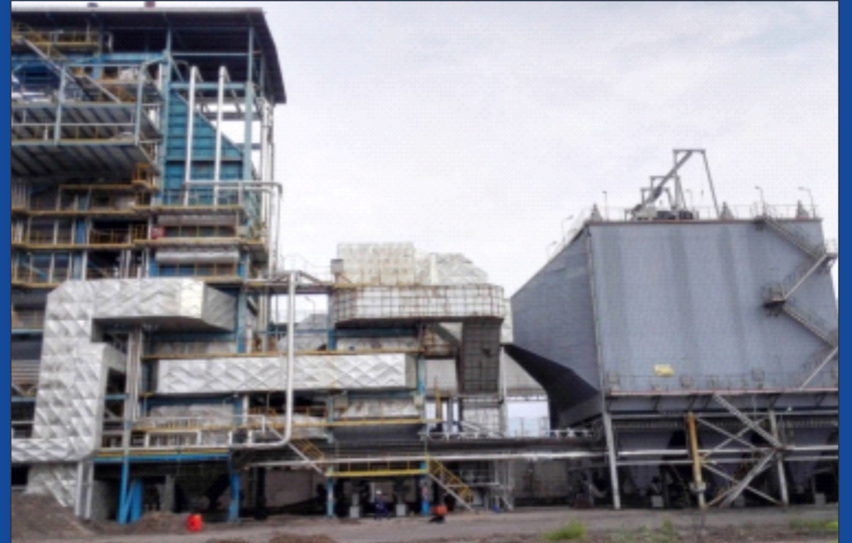
▼ 220 t/h Bagasse Boiler in KKSP, Thailand
