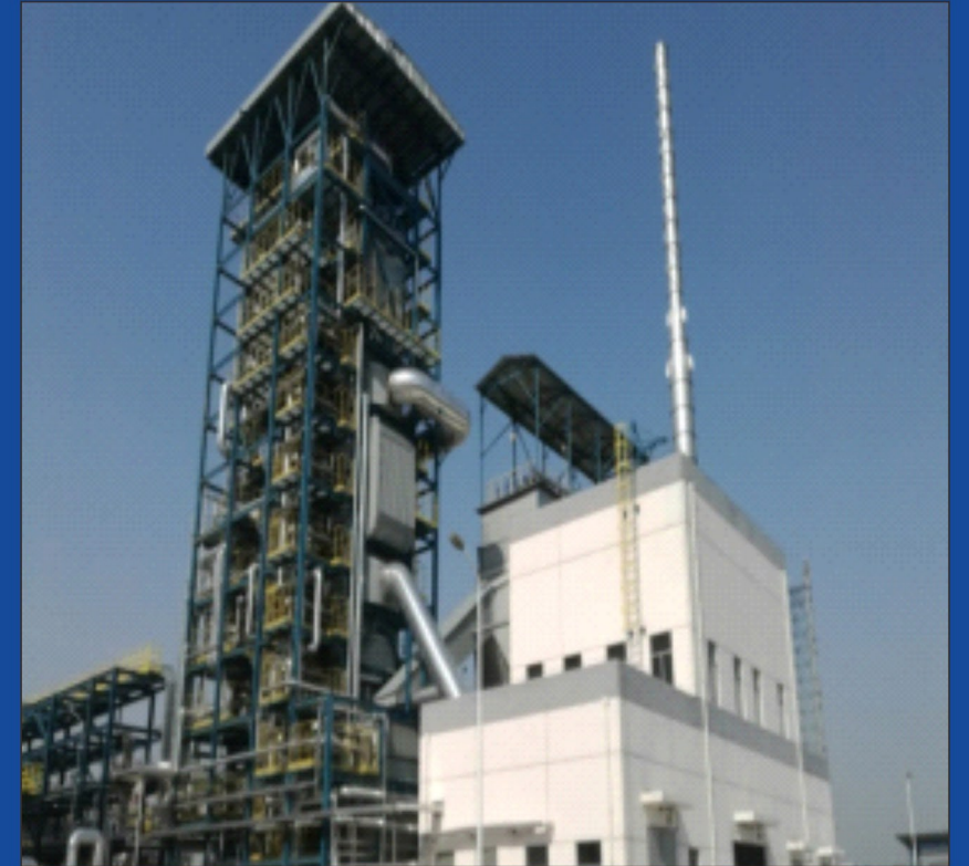
Waste Liquid Incineration Boiler in Zhongan United Coal Chemical Co., Ltd
