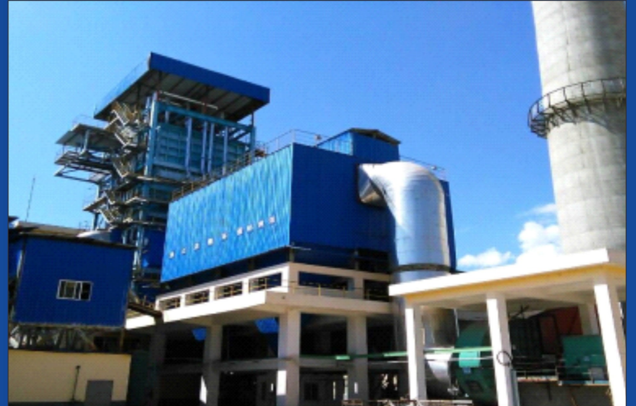
▼ 85 t/h Bagasse Boiler in Yunnan Yunxian Xingfu Sugar Industry Co., Ltd, China
