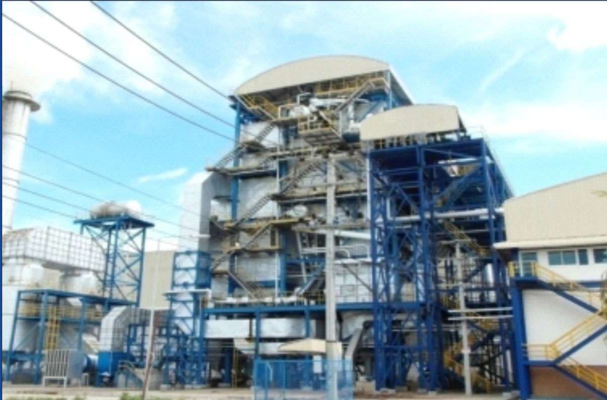
▼ 85t/h Bagasse Boiler in Buriram, Thailand
